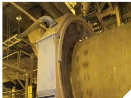
Protecting the gear with a pressurized guard
