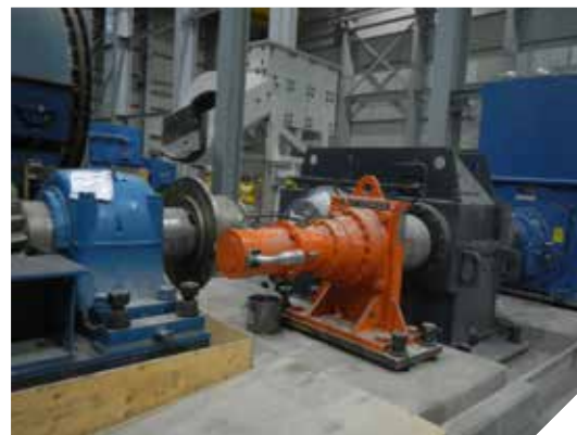
An inching drive through a reducer gear box
