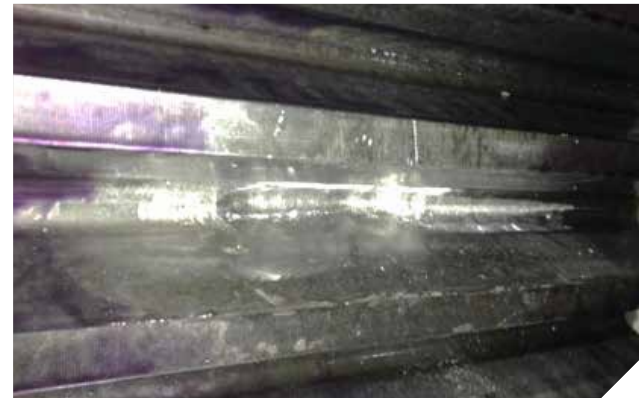
Once detected, cracks are assessed and treated immediately by OEM experts
