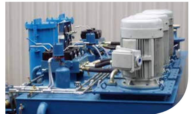
Hydrostatic lubrication system with high pressure pumps
