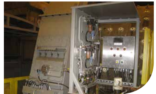
An infrared temperature system tracks the readings continuously
