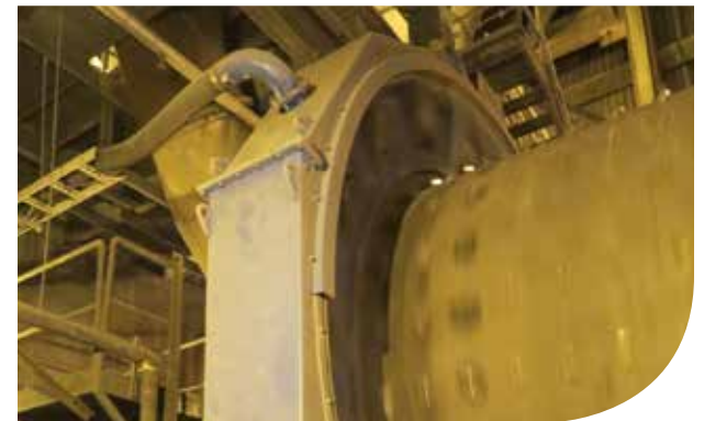
Protecting the gear with a pressurized guard
