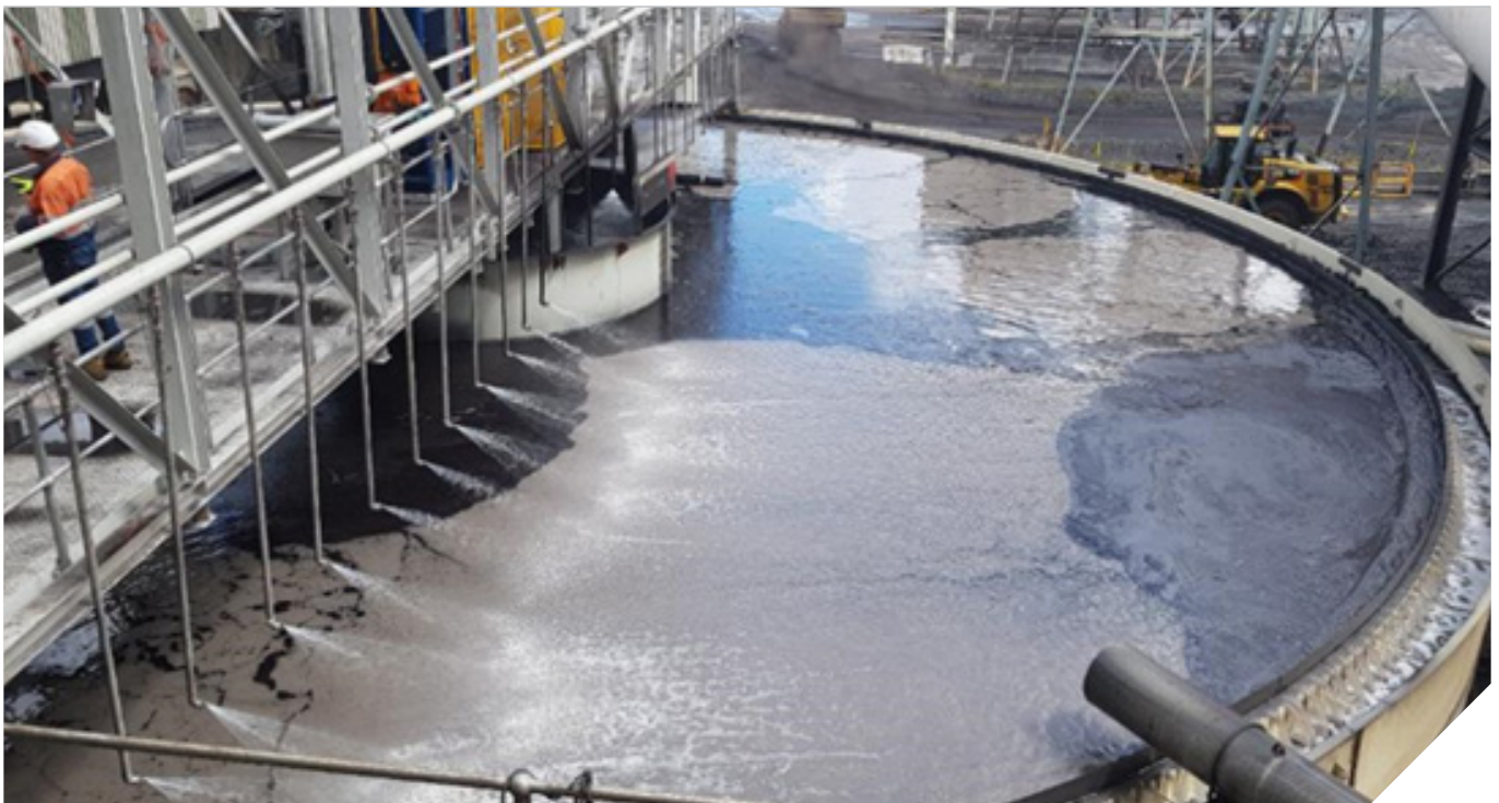
Thickener operating after upgrade, note overflow clarity and low levels of froth on thickener surface.
